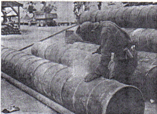
Empty oil drums serve a multitude of purposes at our Pacific bases, such as being welded together for culverts as this Seabee is doing
