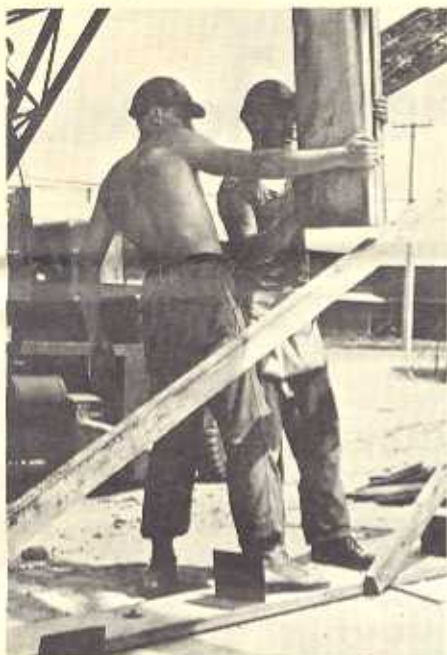
BU3 W.R. Line (left) from Springfield, Oregon, and BU2 L.F. Stark from Erie, Michigan, ease a section of trussed roof into place at the Mag-18 headquarters building.
