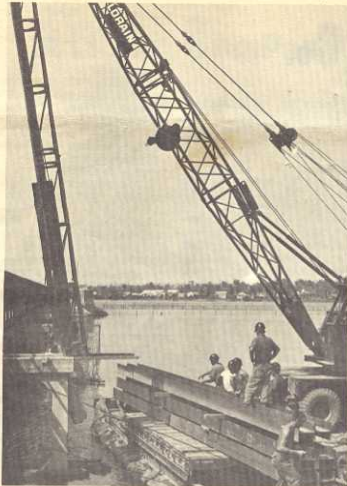
MCB-53's Lang-Co crew place I beams at the bridge site. The men built an H-frame that will be used by an engineering firm to test the strength of the bridge.
