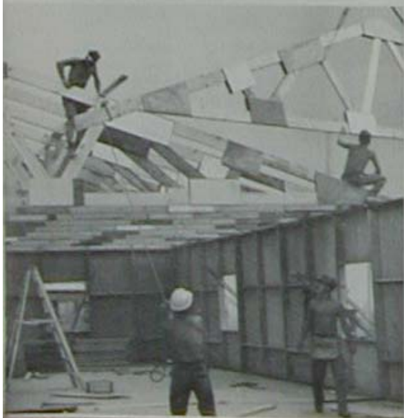
A crew of builders ease a truss into place on one of the Red Cross buildings.
