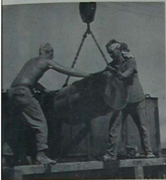
E03 Michael Fennema (left) and EOCN Dennis Casick steady an asphalt barrel before putting it in the plant's melter.
