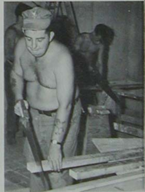
Crew leader BUI R.E. Ousley draws a bead on a 2" X 4" in the Red Cross building while other members of his crew work in the background.
