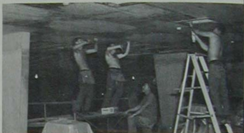
Two builders nail plywood sheets to a 2" X 4" lattice work in the bowling alley while another crew member checks the fit of an air conditioning duct. The entire ceiling was hung from purlins in the Butler building structure.
