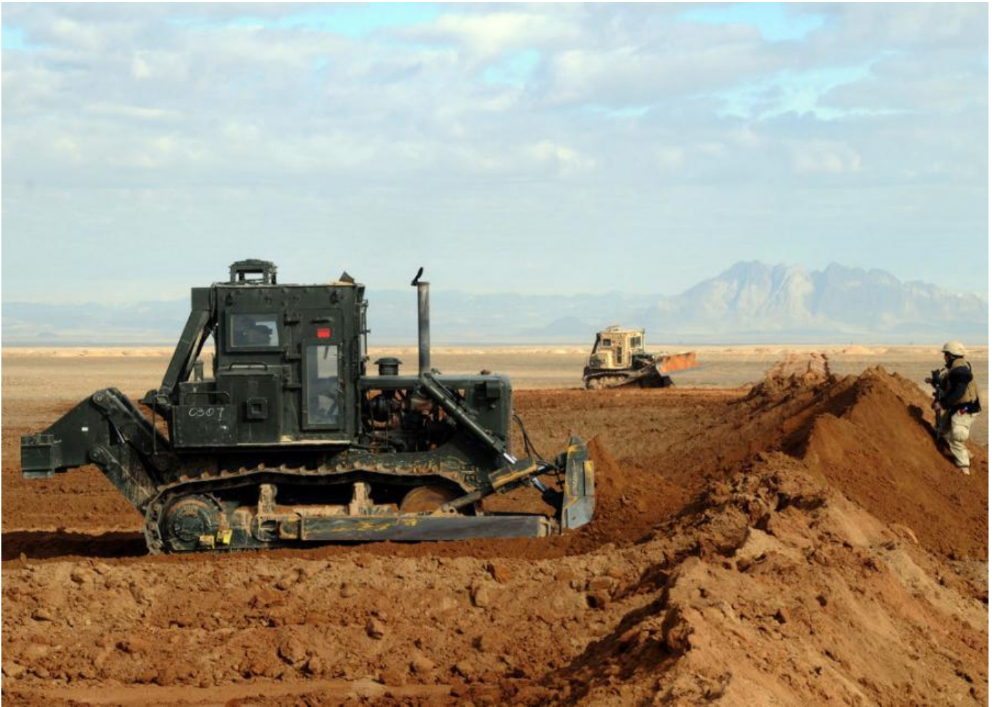
Seabees assigned to Naval Mobile Construction Battalion (NMCB) 7 push dirt into protective barriers utilizing up-armored bulldozers at a forward operating base. NMCB-7 is deployed to Helmand Province, Afghanistan to provide contingency construction support to Alliance forces supporting NATO International Security Assistance Forces Jan. 25, 2009. (Mass Communication Specialist 2nd Class Michael B. Lavender/U.S. Navy photo)
