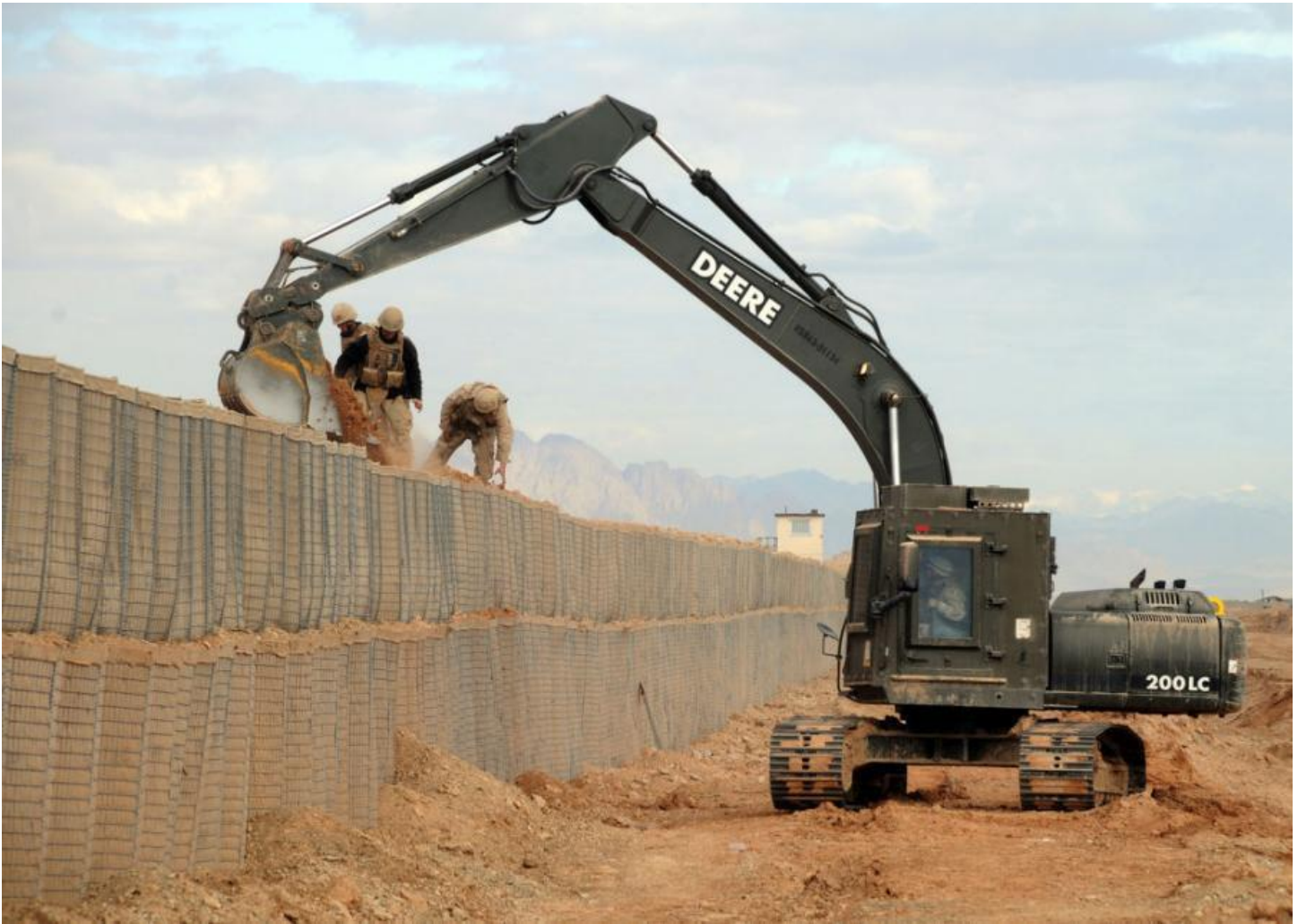
Seabees assigned to Naval Mobile Construction Battalion (NMCB) 7 place dirt into Hesco protective barriers utilizing an up-armored excavator at a forward operating base in Helmand Province, Afghanistan. (Mass Communication Specialist 2nd Class Michael B. Lavender/U.S. Navy photo)
