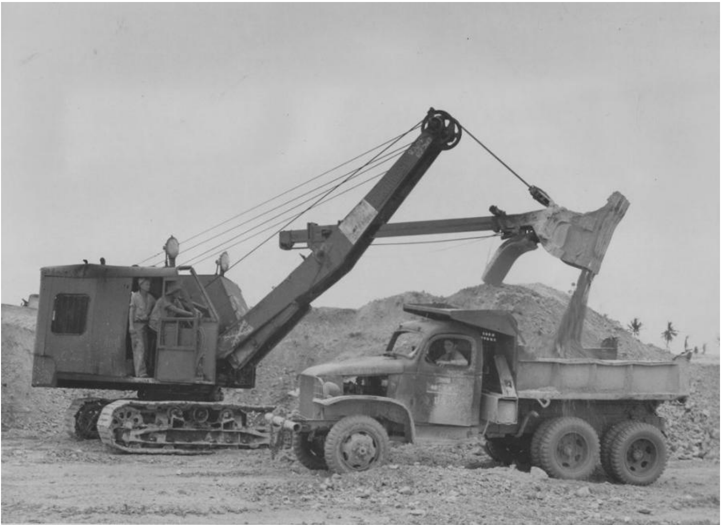
In 1945, Seabees use a 1.5 yd. Northwest Shovel to load a truck with coral. Coral, being readily available, was used as fill, as a subbase for airstrips and a multitude of other uses in the Pacific. (U.S. Navy Seabee Museum photo)
