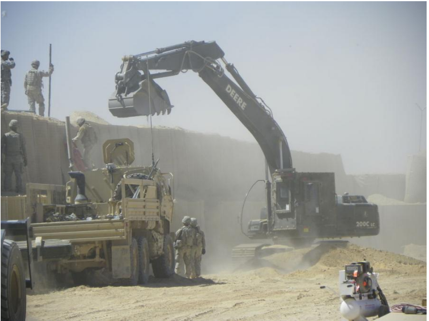
Seabees assigned to Naval Mobile Construction Battalions (NMCB) 40 and 18 and Soldiers assigned to the 101st Airborne Division complete a Hesco barrier at Combat Outpost in Kandalay in Southern Afghanistan on Oct. 8, 2010. The 101st Airborne Division is occupying the combat outpost. (Chief Mass Communication Specialist Leif HerrGesell/U.S. Navy photo)
