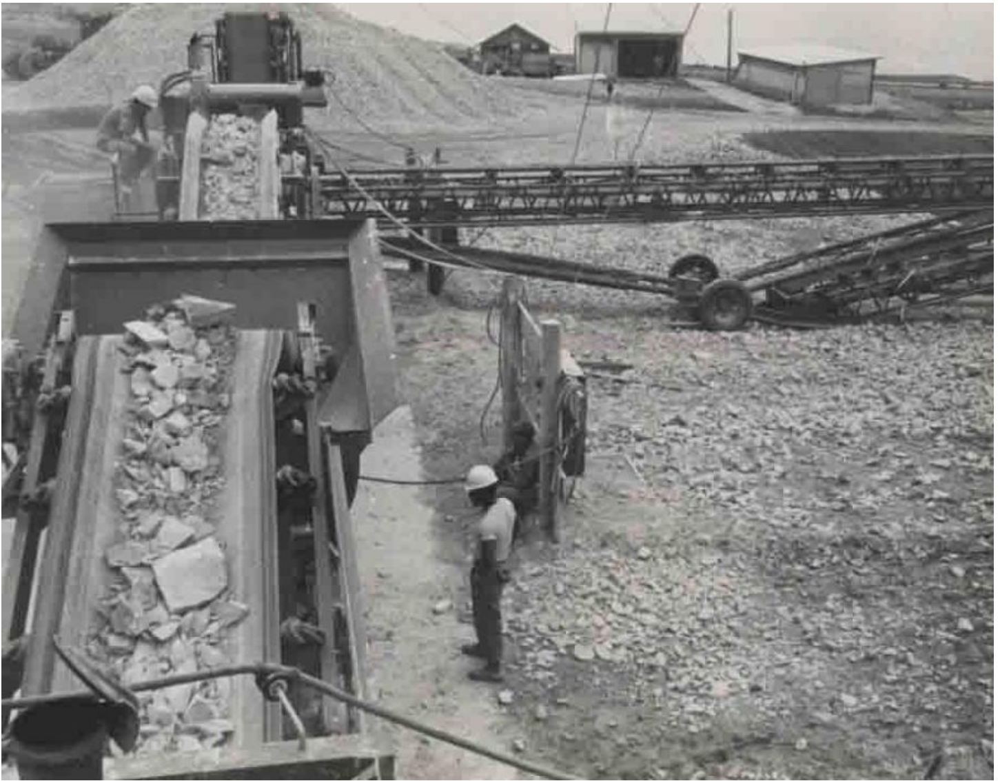
Portions of the rock quarry inside Camp De Shurley being worked on. (U.S. Navy Seabee Museum photo)
