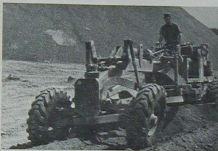
E0C G.R. Sutton From Colfax, Illinois, puts a grader to work at F-Company's rock crusher site.
