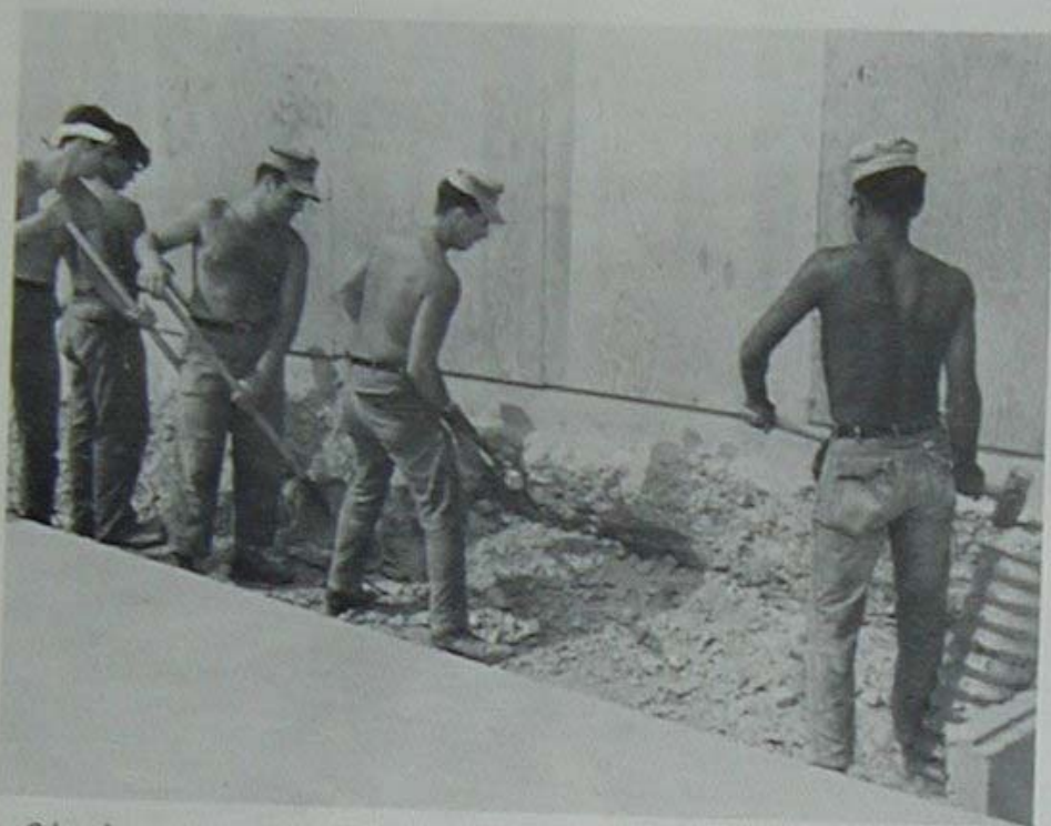
Digging a form for a concrete drainway at FLC are (l-r) BU3 Edward Swiski from Hatboro, Pennsylvania; BU3 Garrit Zwakenberg from Cave, Kentucky; BUCN Peter Uzzardo from West Mount, Illinois; BU3 Ronald DeRonde from Cincinnati, Ohio; and CN Stan Walker from Nome, Alaska.
