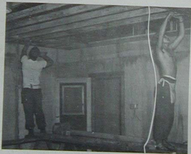
Nailing in joists at the Data Processing facility are BU2 Henry Baldinger (back to picture) from Clifton, New Jersey and BU3 Gerald Pellecchia from McKeesport, Pennsylvania.
