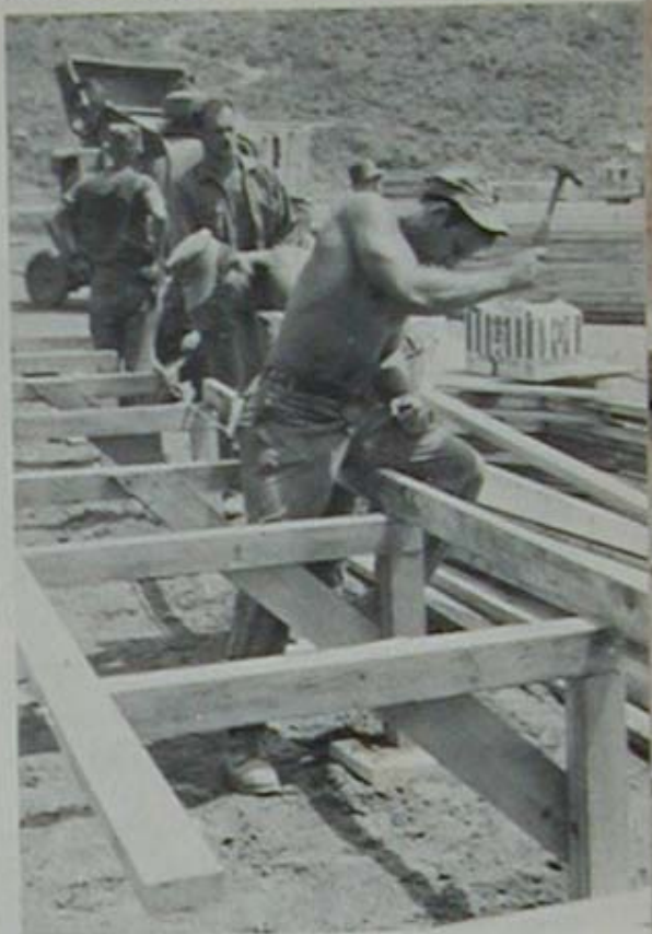
Crew members construct the SEA huts they will live in while on the jobsite
