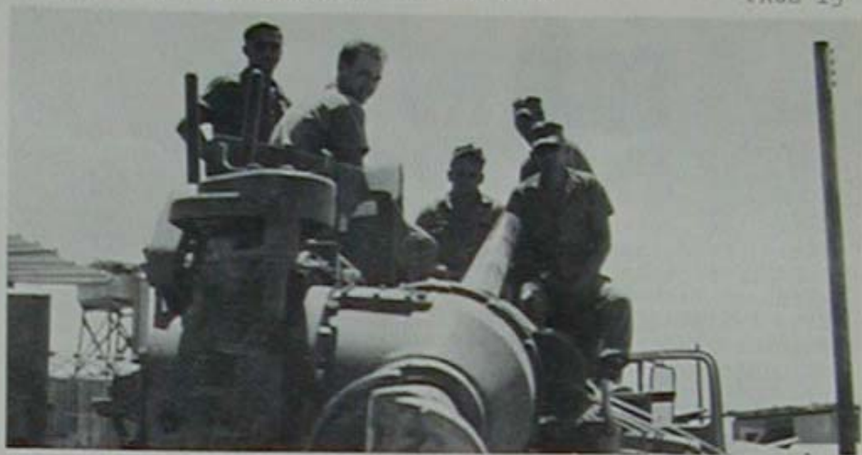
Bravo Company line truck--(left to right) Gilbert, Mull, Hubbs, Hutcheison and Berg drill holes for telephone poles.
