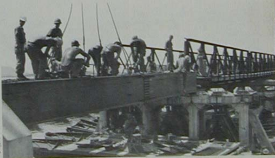
A crew sets the heavy steel H-beams in place for the first span. The one lane French bridge with its high railing is in the background.
