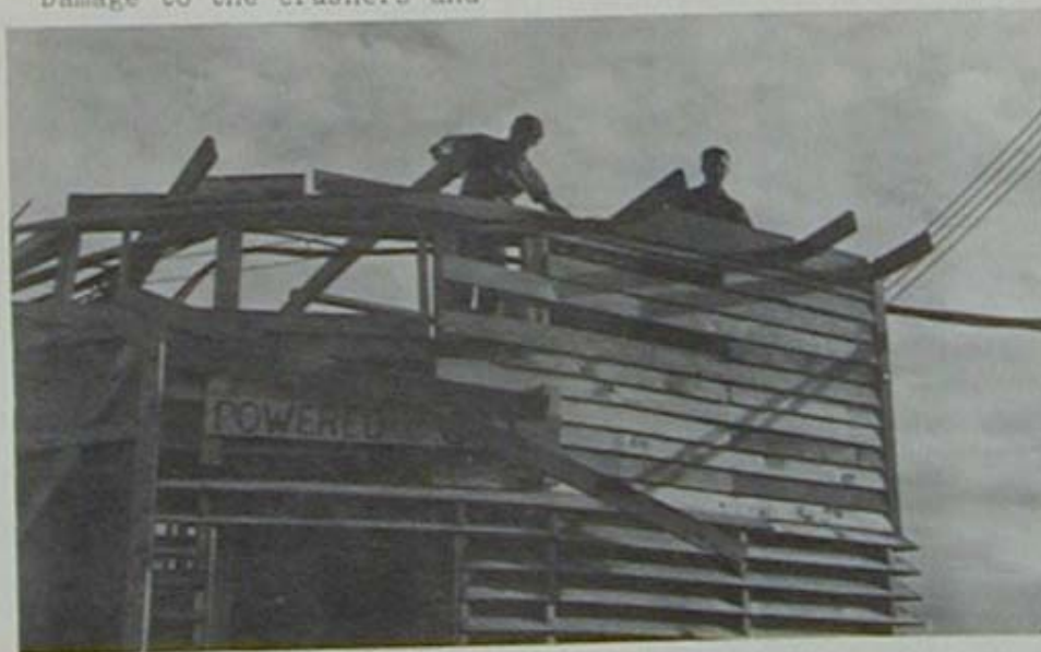
E03 Robert Trammel (left) and E0CN Roger Schultz clear wreckage at the generator shack.
