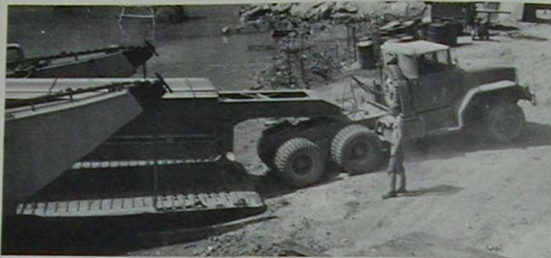
A ten ton truck carrying steel beams disembarks from the LCU that brought it from Da Nang to the bridge site.
