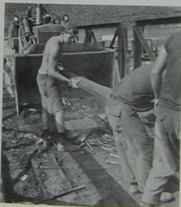
Splinters fly as these MCB-53 Seabees rip up the old French decking.
