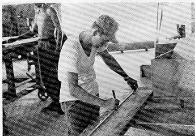
BUL3 R.A. PETERS, "D" CO., of Haverhill, Massachusetts laying out shelving for Utilities Shop.
