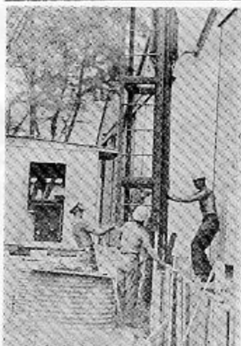
Members of Delta Company steady pile-driving leads as they work at the site of the new Combat Operations Center at the 3rd Marine Amphibious Force camp.
