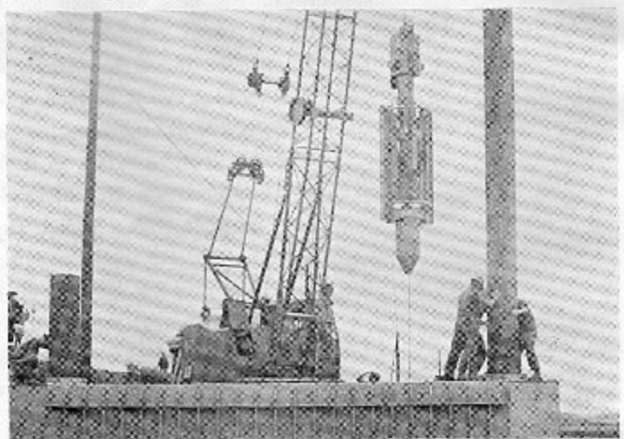
The construction Seabees of 53 center a pile in an Ammi Pontoon "spudwell" during the bridge's erection.
