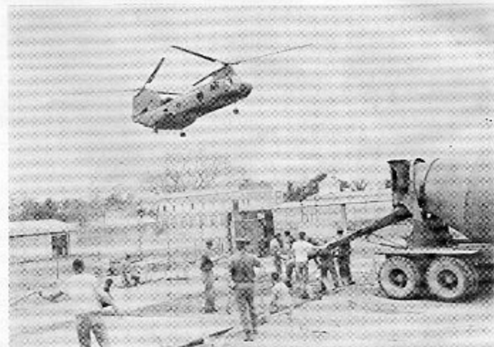
Delta Company "Devils" are temporarily distracted from their concrete pouring for the new Marine barracks at the III MAF as a CH-46 helo hovers above them.
