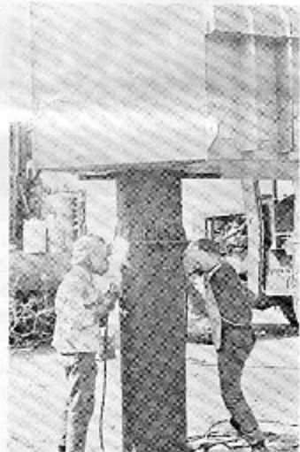
Seabees from 53 weld the retaining rings on support piles during the construction of a new Ammi Pontoon Bridge near DaNang. The retaining rings are used to suspend the pontoons above the water.
