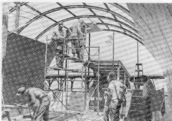
Members of "Charlie" Company shown in the process of constructing a Quonset hut which will be used for storage purposes at the NSA Hospital in DaNang East.
