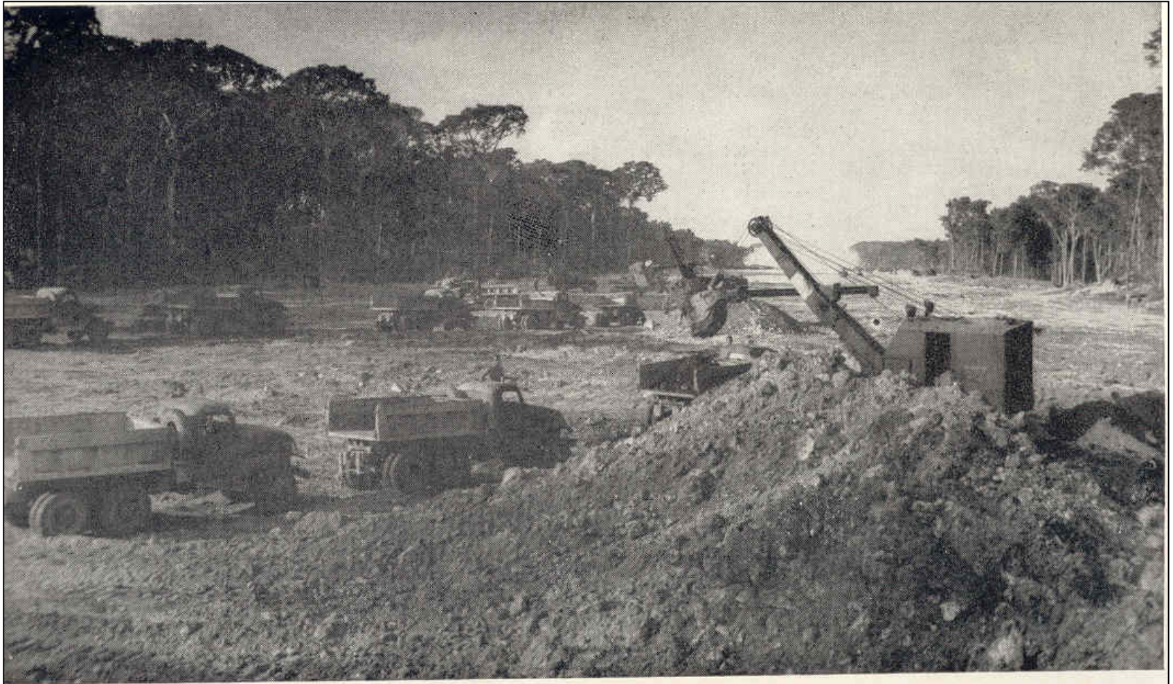
2. Removing the windows of earth piled up by the bulldozers — fourth day. (Official U. S. Navy Photo)
