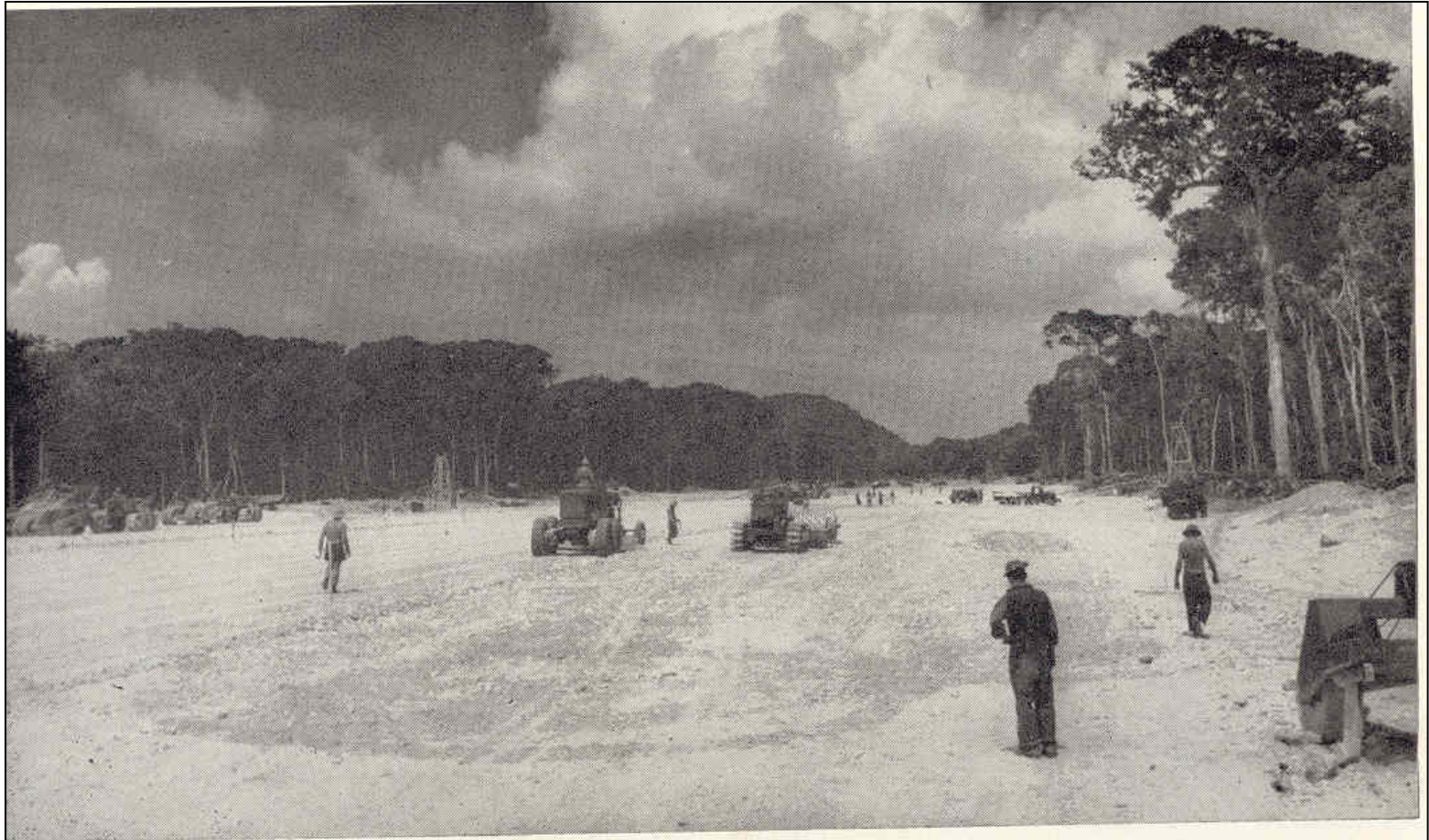
4. Grading and rolling with the "sheeps's foot" roller – eighth day. (Official U. S. Navy Photo)
