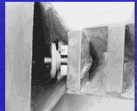
Wedge, bolt, and nut attachment employed between pontoon corners and angle stiffeners
