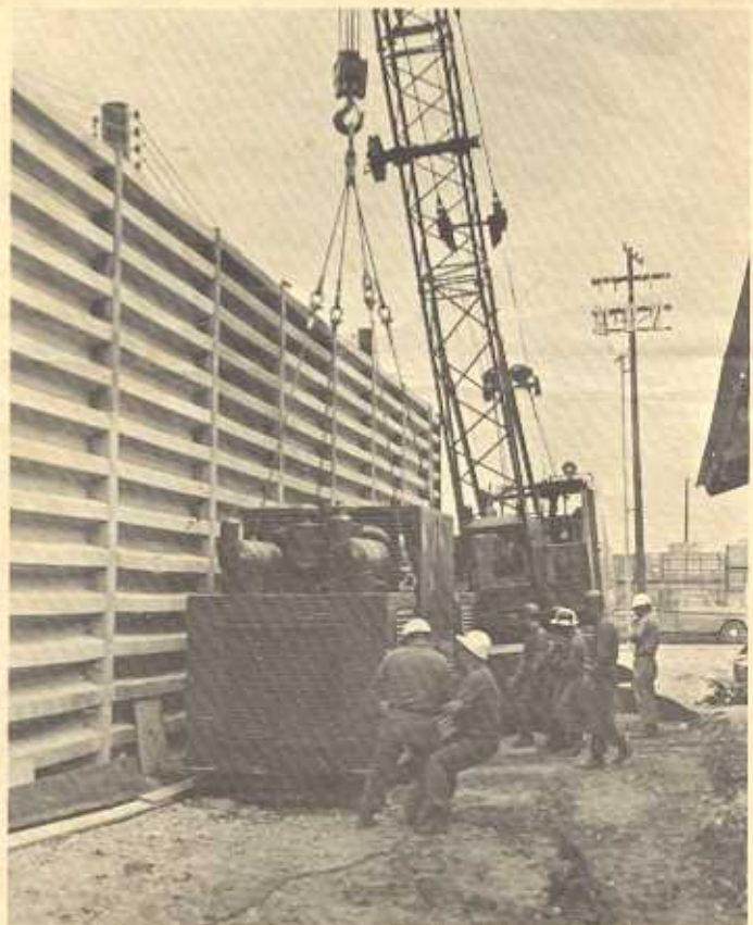
MCB-53 Seabees, with the aid of a crane, put a generator in place that will be used for the Data Processing facility.
