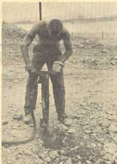
BU3 L.M. Dennis from Columbia, South Carolina, breaks up the ground at the bridge site with a jackhammer. In the background is what remains of the old Liberty Bridge.
