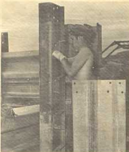
BU3 Richard Boyce (center) from Newcastle, Delaware, and SW2 Bill Ward (background) from Harrisburg, Pennsylvania, tighten down revetment brackets during the construction of a computer facility.
