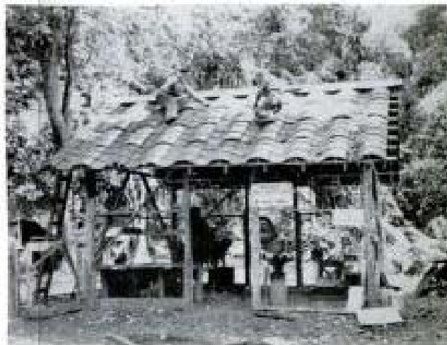
Improvisation and ingenuity go hand in hand wherever the Seabees take hold, as this tin roof in the South Pacific shows. It is made of partially flattened gasoline drums
