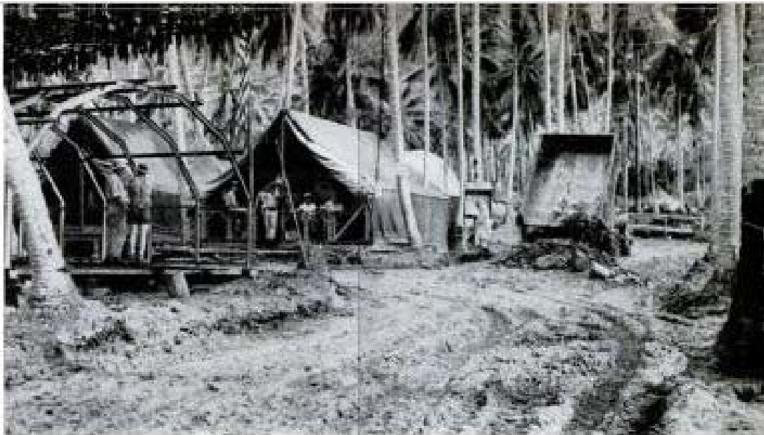
Mud and jungle fail to halt the Navy's Construction Battalions. Here Seabees dump rock from a beach to harden the soft New Guinea soil for road building as others in the outfit erect shelters
